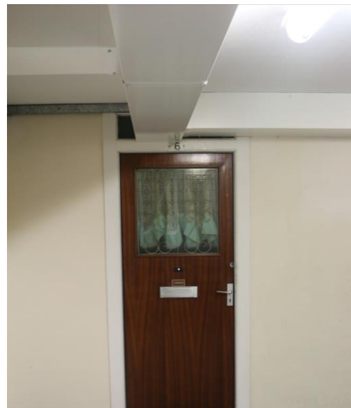
Figure 27: Flat door and DH piping
