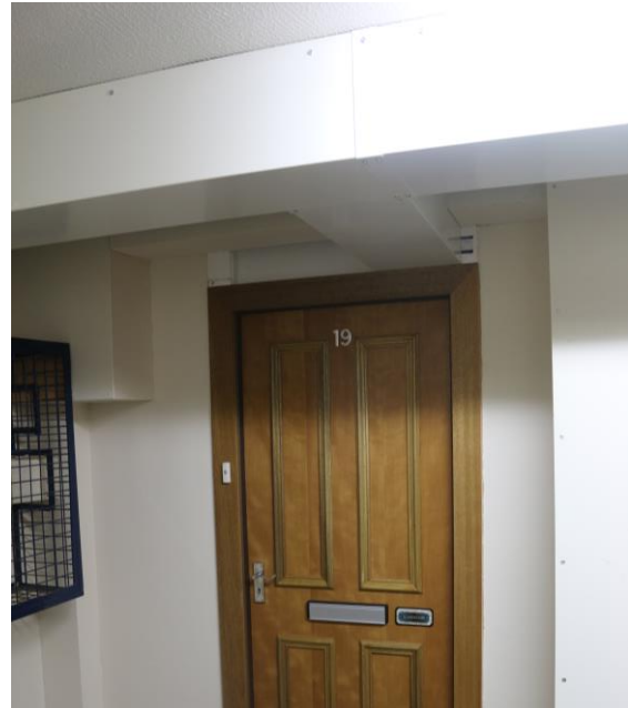
Figure 19: Flat door and DH piping
