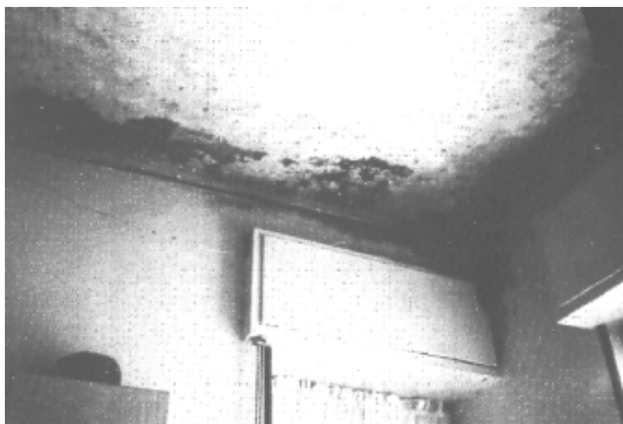
Figure 6: Mould growth in the monitored house.
