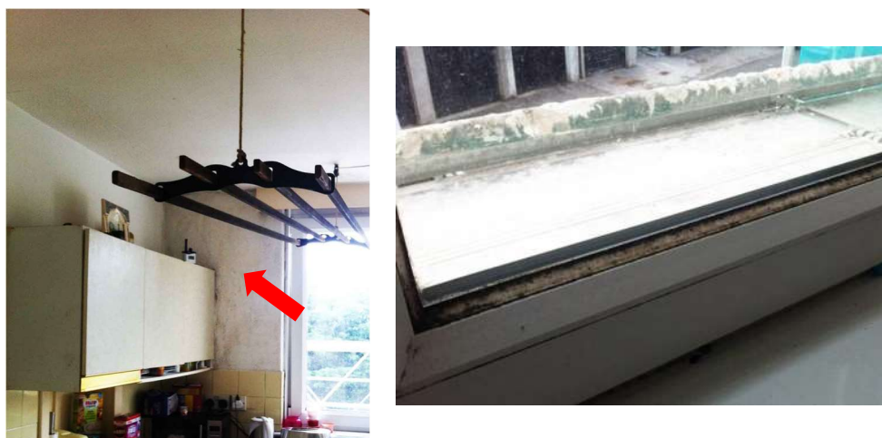
Figure 7: Occurrence of a severe mould growth problem.
