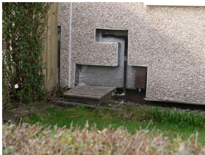
Figure 8: thermal bridge due to non-insulated section around a gas pipe and meter box.
