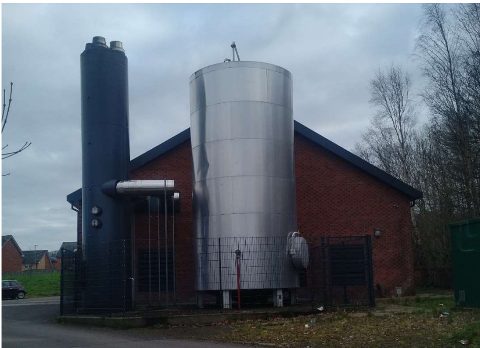
Figure 6.2: WWHC hot water tank and flue chimney in foreground, and boiler house in background
