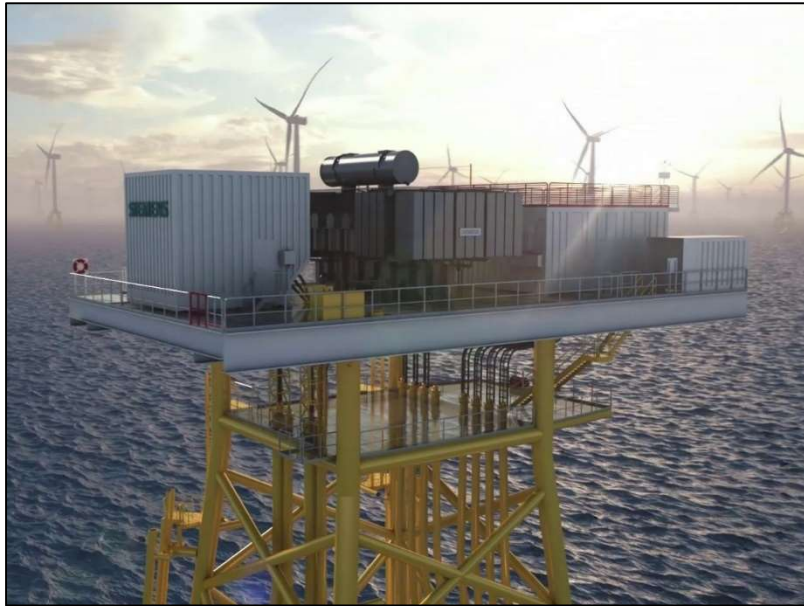
Figure 21: Offshore transformer module for Moray East wind farm, where output voltage from the wind turbines will be transformed from 66 kV to the transmission voltage of 220 kV [93].
