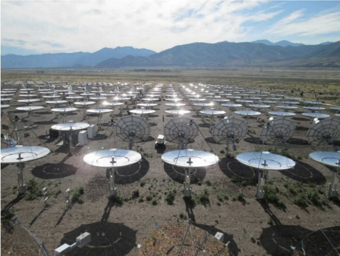
Figure 12 Tooele army depot solar dish/engine CSP plant (source: https://galvanizeit.org/project-gallery/stirling-solar-array-tooele-army-depot )
