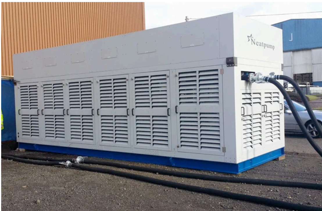
Figure 6: Example of the ASHP deployed at Hillpark Drive DHN (Pearson, 2015)
