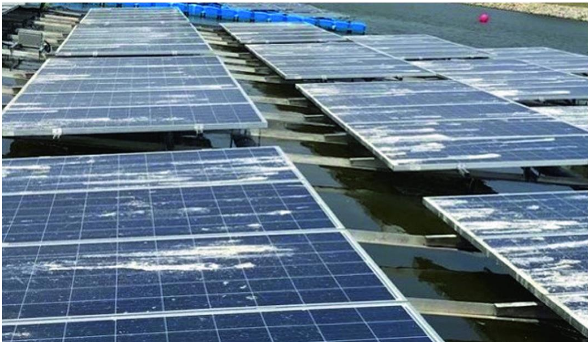
Figure 21 - Bird Soiling at Sheplands Floating Solar Plant
