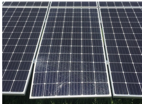
Figure 7. Image showing deformation of the panel due to mechanical forces. Picture taken in PV park used for the case study in Pärnu, Estonia.
