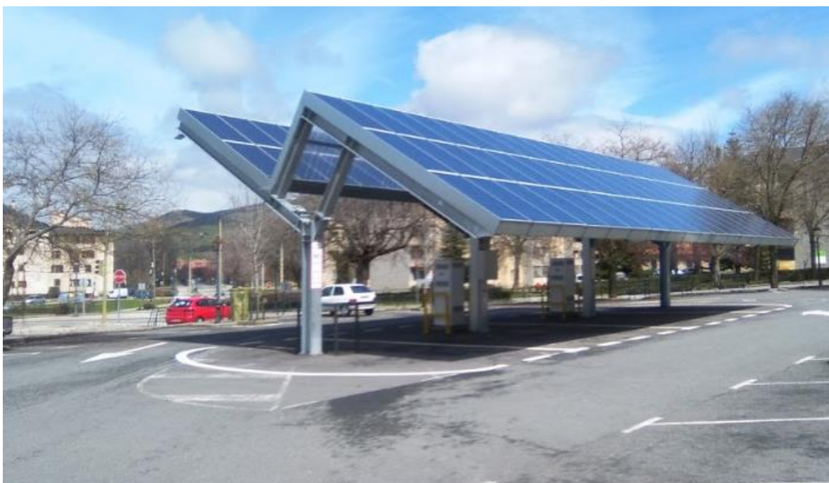
Figure 2: Photovoltaic Electric Vehicle Charging Station.
