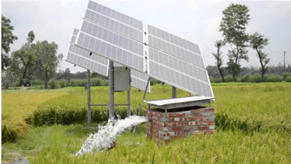
Figure 5: Example of solar irrigation. [20]
