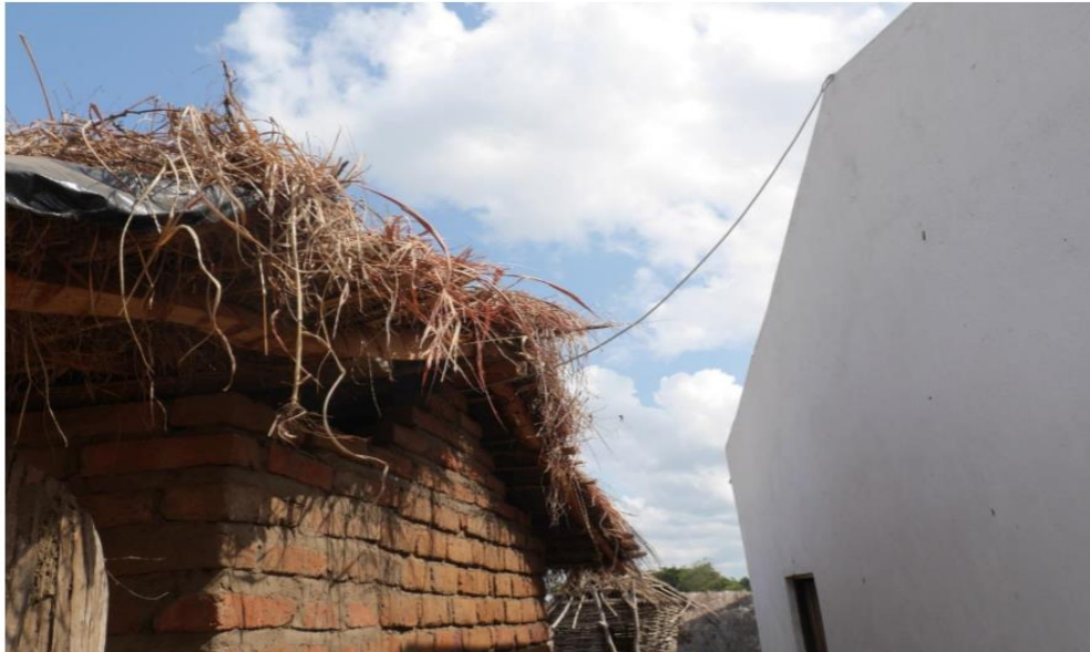
Figure 3: Example of an unofficial connection in a rural community. [6]
