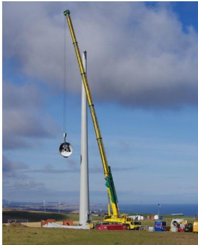
Figure 23: Photograph of construction of one of three 77 m wind turbines at Easter Melrose, Aberdeenshire (© Orkney Sustainable Energy Ltd. 1995 – 2019)
