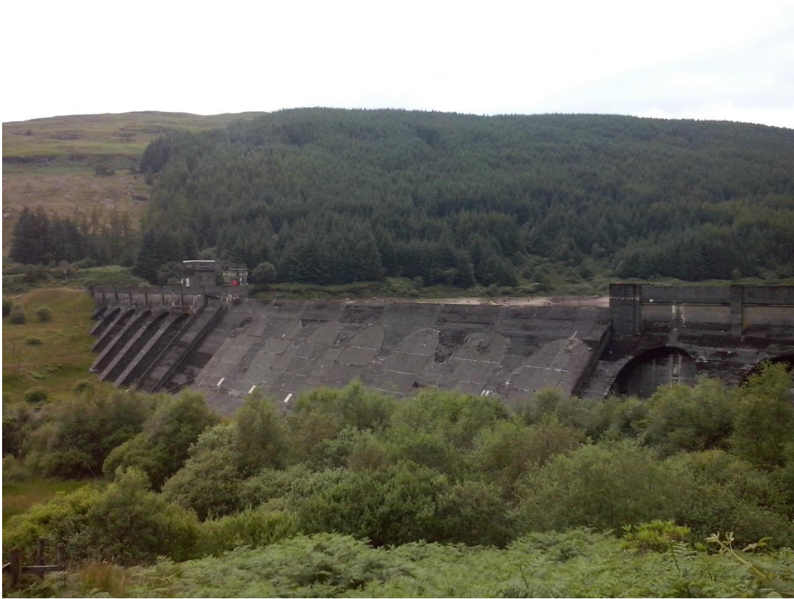
Figure 1: Author's photograph of one of two dams built in 1953 creating Loch Tarsan on the Cowal Peninsula, a 12,500,000 m 3 reservoir (Argyll and Bute Council, 2014) feeding Striven power station
