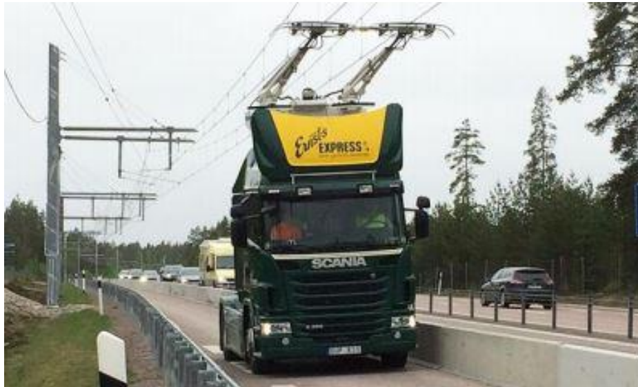
Figure 17: Overhead Catenary Charging System
