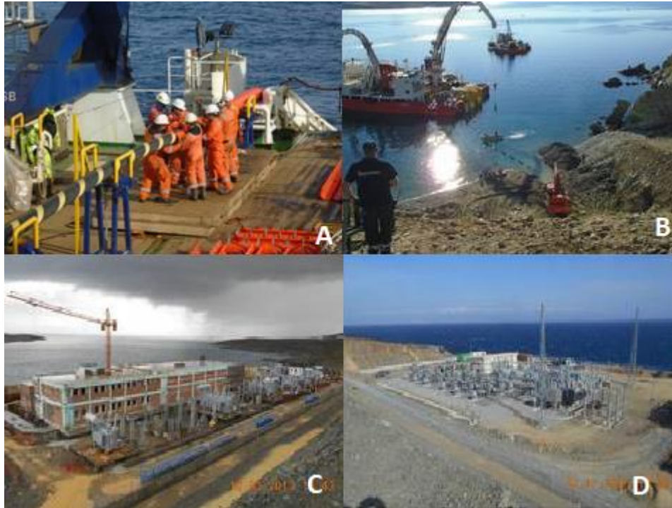
Figure 8: Construction works from Phases A, B, C, D of Cyclades islands connection to mainland's grid
