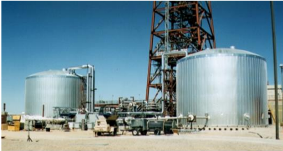
Figure 35: TS Tanks from the Solar Project (Bradshaw, et al., 2002)
