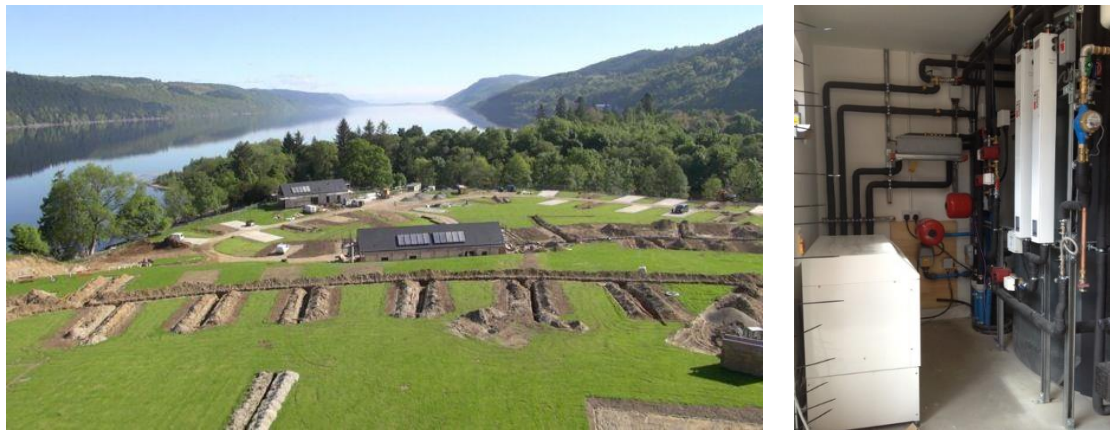
Figure 14. Loch Ness Shores Foyers Camping Site in Foyers; district heating construction process (left), successfully installed heat pump system (right) (Kensa Heat Pumps, 2017)
