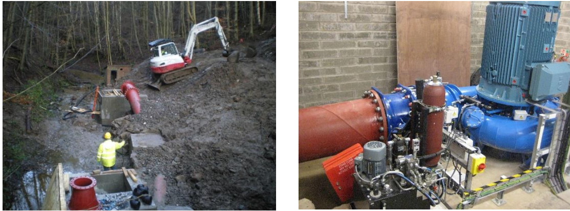
Figure 24. Harlaw micro hydro project in Balerno; construction phase (left) and installed Francis turbine with other mechanical and electrical equipment (right) ( Harlaw Hydro, 2017 )
