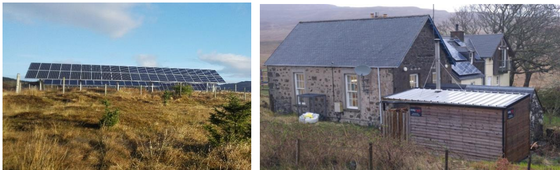
Figure 27. Solar PV panels on the Isle of Eigg; community owned PV array (left) and PV panels installed on the roof of the primary school (right); pictures taken during a field trip on April 4, 2017
