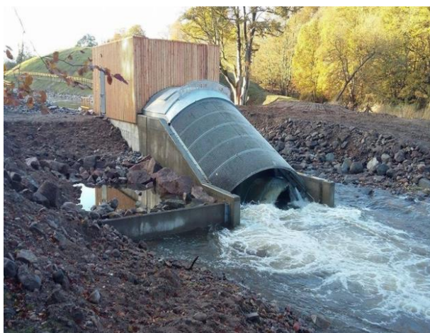
Figure 22. Archimedes Screw as a part of Donside Hydro Community project (Power-Technology, 2017)
