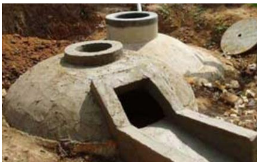
Figure 2.1. Small-scale digester in Uganda (Source: Community by Design)
