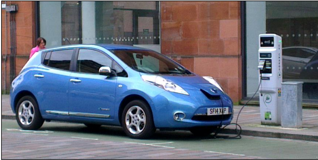
Figure 4 EV Charging Point in Glasgow (McAllister, 2015)
