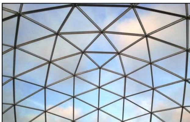
Figure 41: View of the sky through the transparent glass cover - The Nature House, Norway (Solardome Industries)
