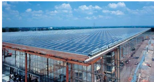
Figure 49: Solar panels on the roof of Mont Cenis Academy (Education Academy Mont-Cenis)
