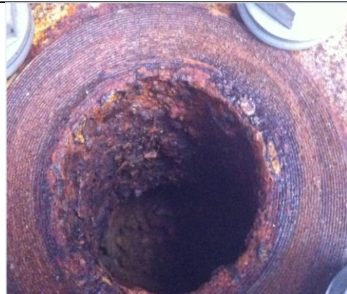
Figure 31 Cooling Water Isolating Valve Close Up
