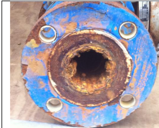
Figure 30 Cooling Water Isolating Valve
