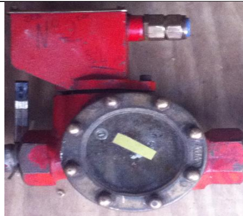
Figure 29 Cooling Water Flow Control Relay
