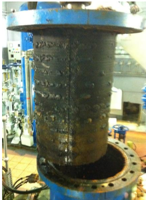
Figure 27 MIV Control Water Rotary Filter
