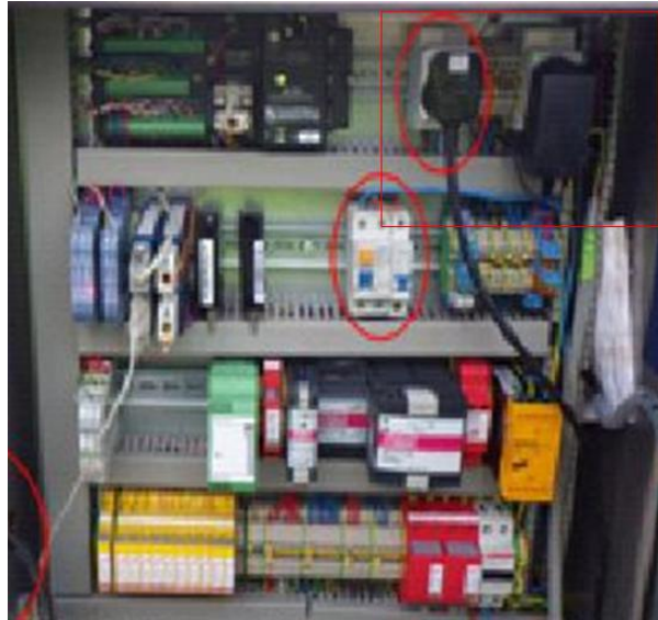
Figure 13: Onsite Power Supply for LIDAR
