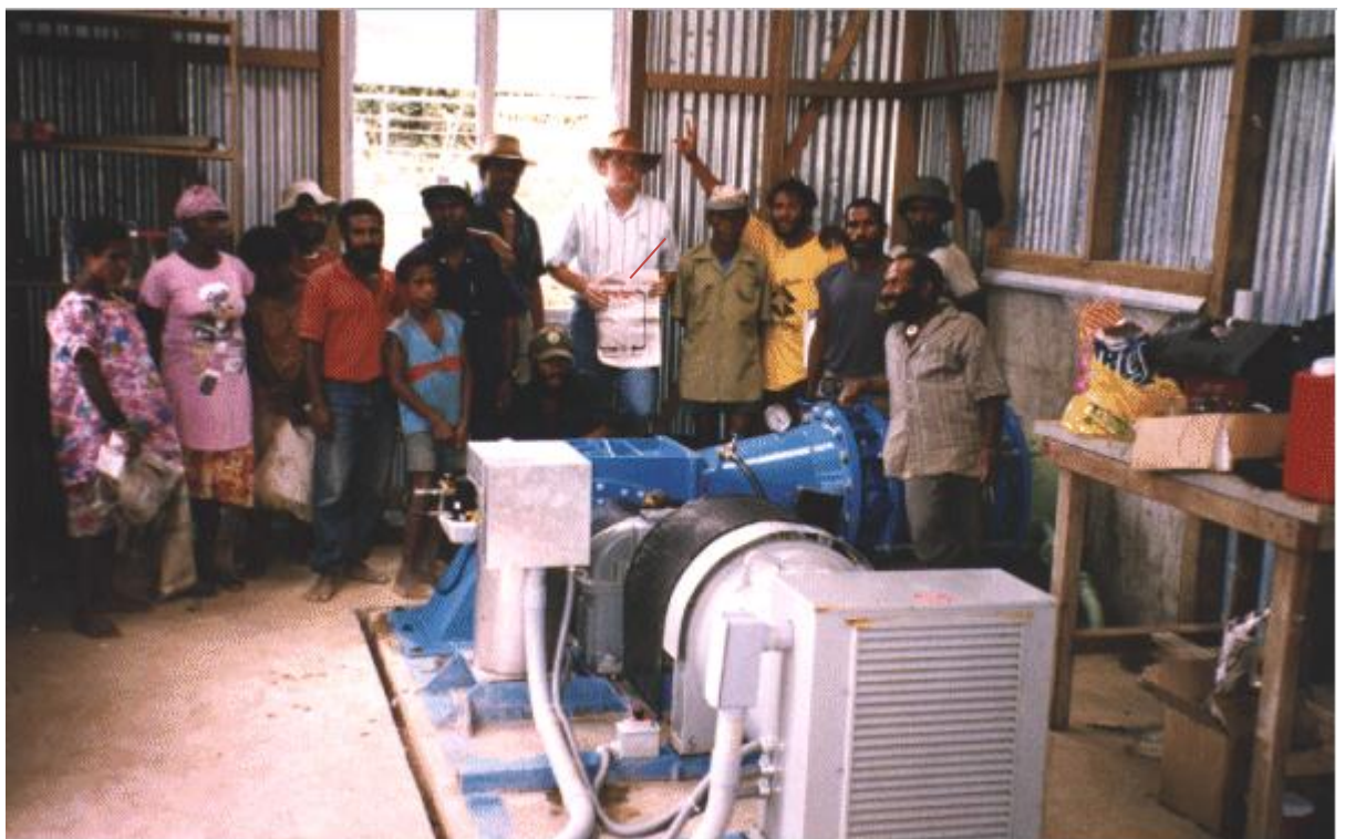
Fig 5,6 An example of a 100kW cross flow turbine system in a remote school in Papua, New Guinea.
