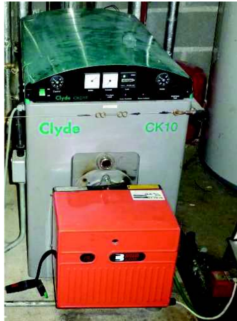
Figure 5-2: DHW Oil Boiler
