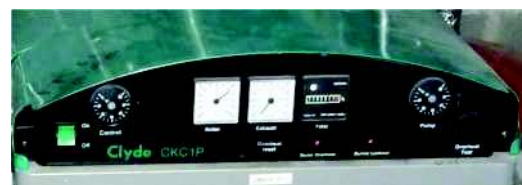
Figure 6-10: Oil Boiler Control Panel
