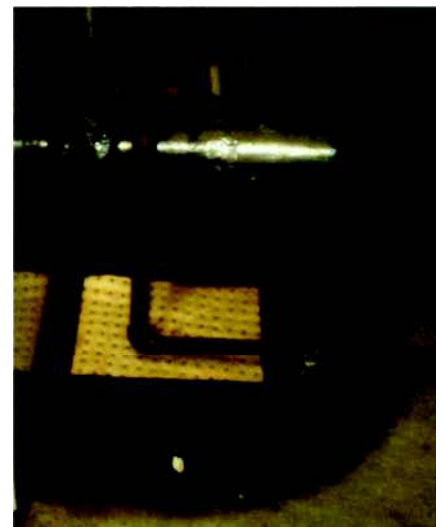
Figure 6-1: Potential Oil Leak
