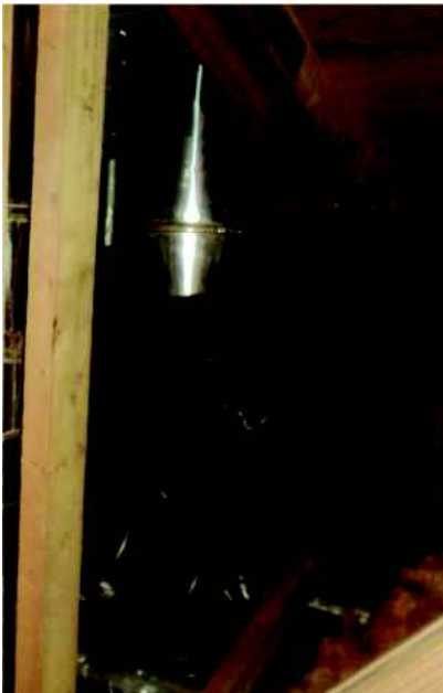
Figure 6-8: Bend in Flue above Plant Room
