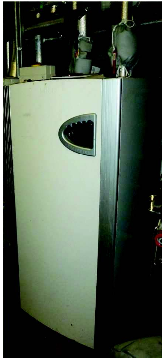
Figure 5-1: DHW Heat Pump (HP 3)
