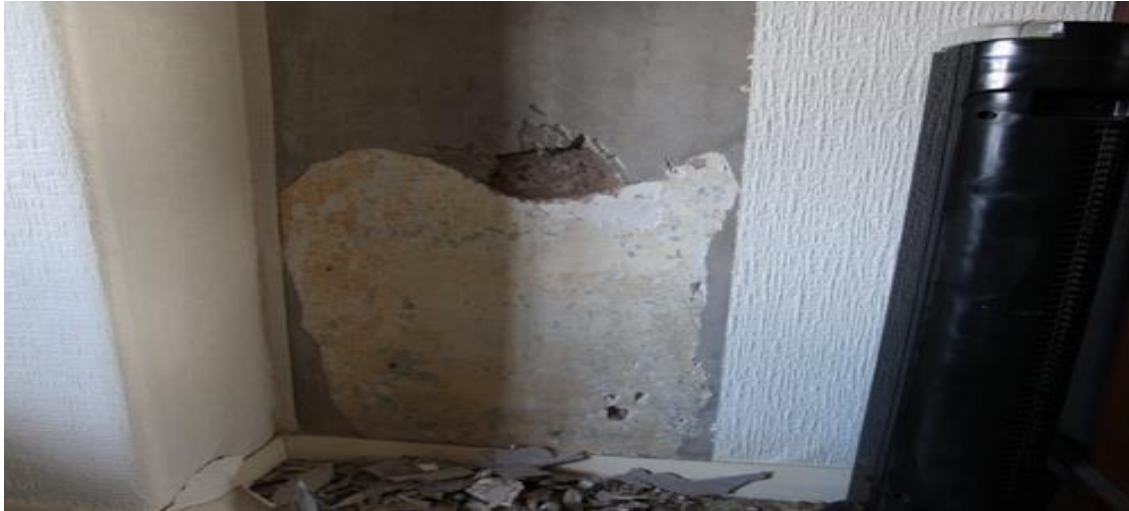
Figure 2: Condensation on walls [65]
