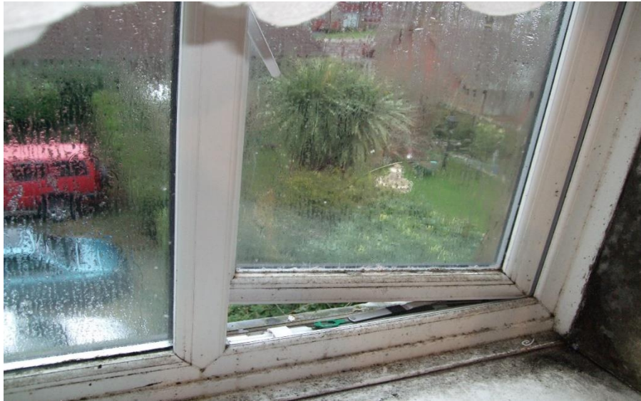
Figure 3: Mould growth on windows [66]
