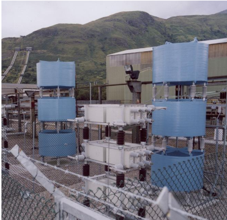
Figure 2-10: Air-Core HVAC Shunt Reactors (National Grid, 2010)
