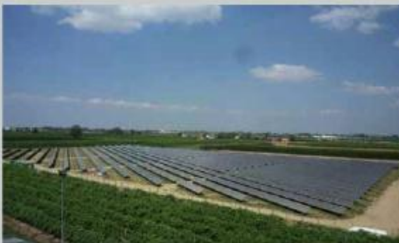
Free-field installation, Italy
