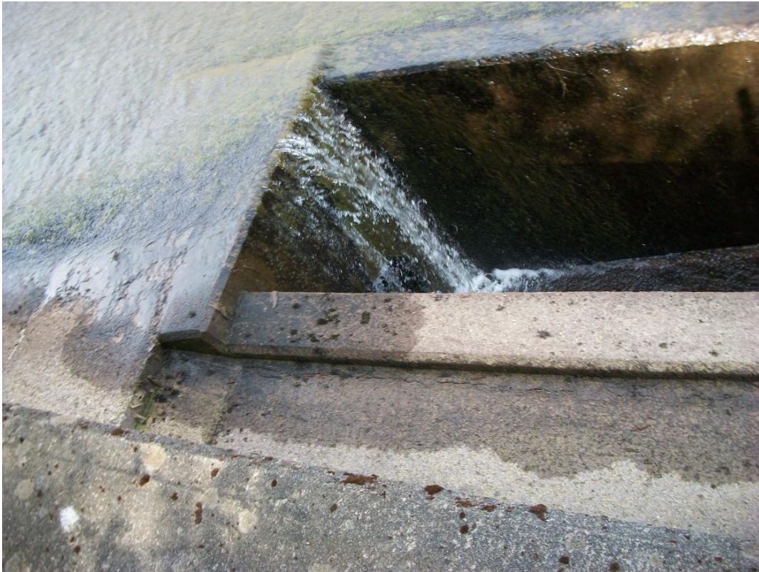
A-3: Scour valve exit
