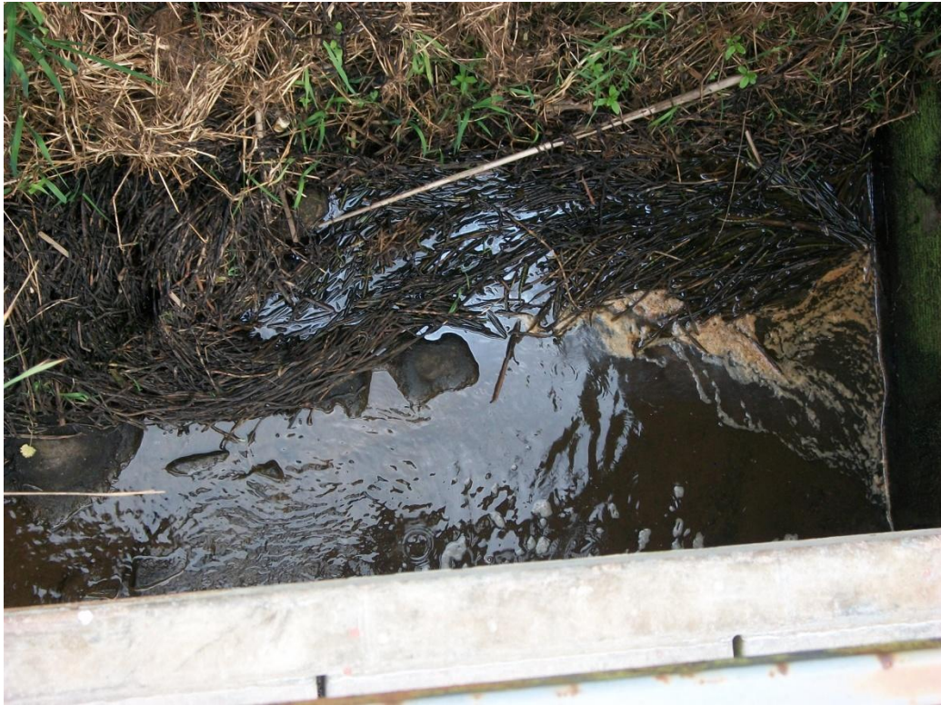
B-3: View of high levels of debris, grass and mud in water
