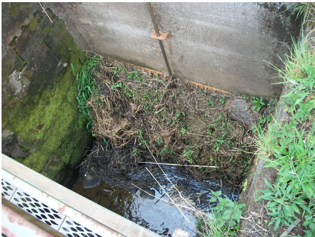
B-4: Debris blocking entrance to culvert
