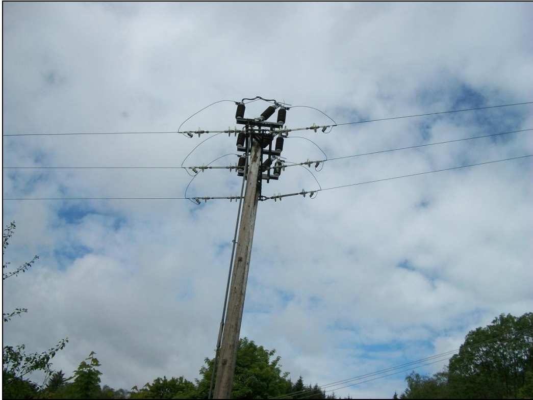
Figure 26: Three phase 11kV line that is local to Bishops Glen reservoir
