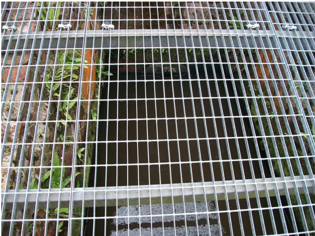
B-6: Just visible is culvert exit sitting below the water line
