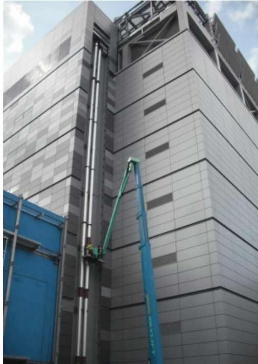
Figure 17 – Communications centre with external water pipes (Searle-Barnes, 2010)
