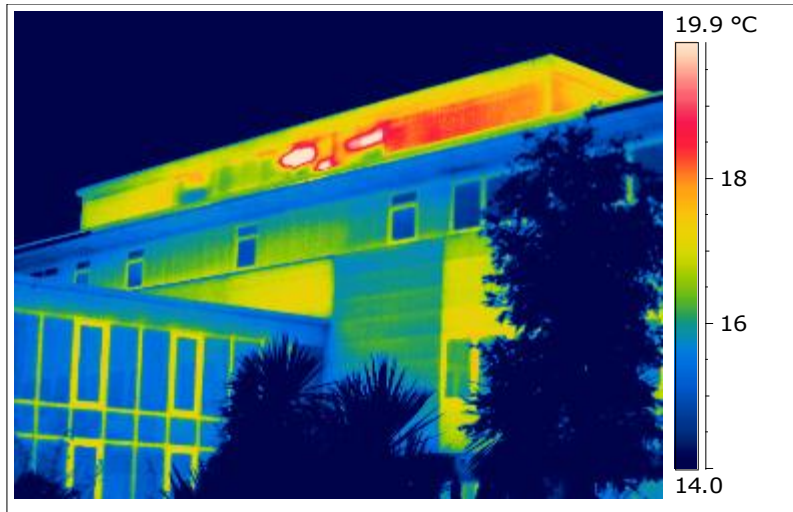
Figure 17: Thermal image of AHU during the bank holiday
