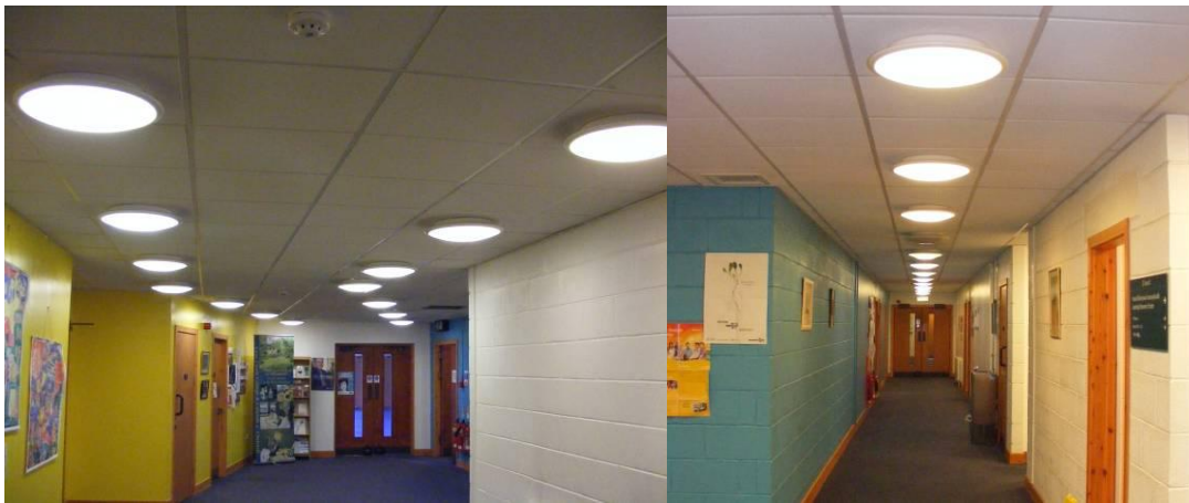
Figure 25: Images of excess lighting in the Facilities Building
