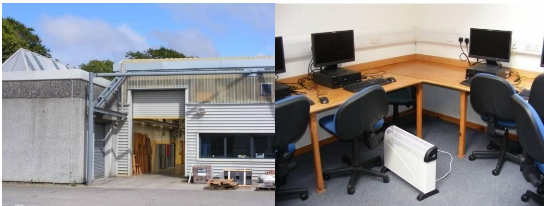
Figure 13: Engineering Building glass/fibreglass roof (left) and use of electrical convective heaters (right)
