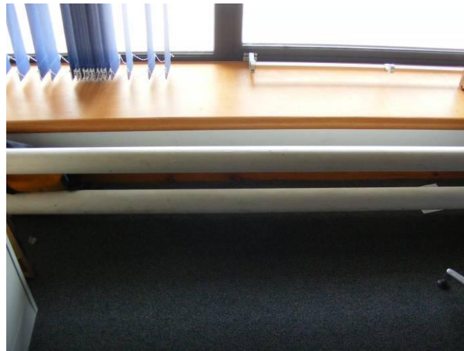
Figure 14: Heating pipe running along the upper floor of the Rural Building
