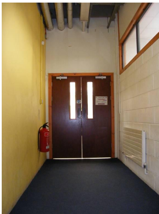
Figure 26: Image of doors leading from Facilities Building to Engineering Building. Gap from floor to bottom of door is 15mm
