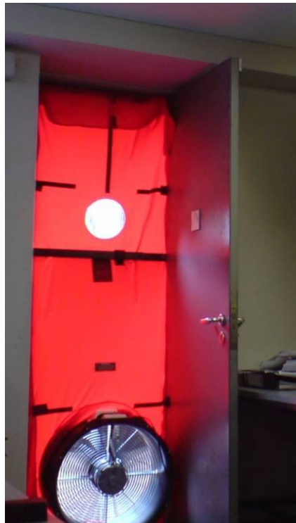
Figure 5: Set up of the air pressure testing kit on the classroom E005 in Engineering Building
