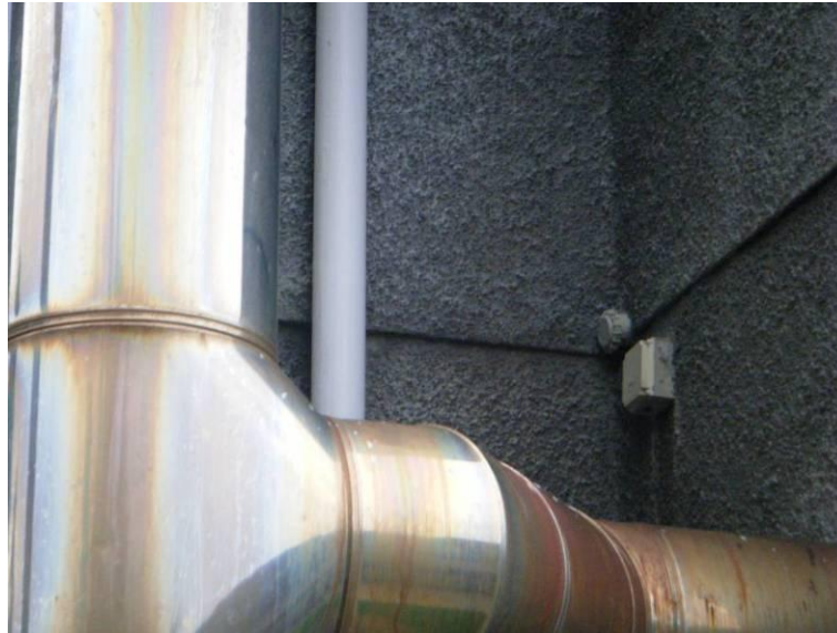
Figure 9: Outside temperature sensor situated too close to flue exhaust pipe from boiler house
