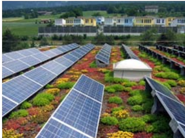
Figure 15: Green Roof with Photovoltaic Panels [5]
