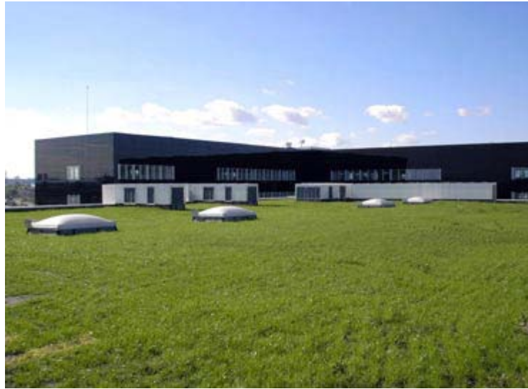
Figure 5: Extensive Green Roof (Prague, Czech Republic) [5]
