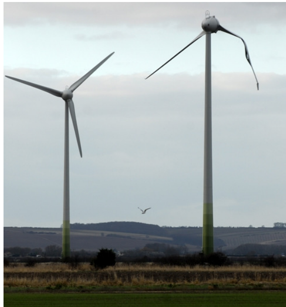
Fig. 3.7: Wind Turbine with both a damaged blade and a missing blade (Source: [22])
