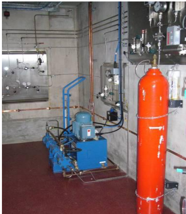
Figure 6 - HARI Diaphragm Compressor and Buffer Tank [11]
