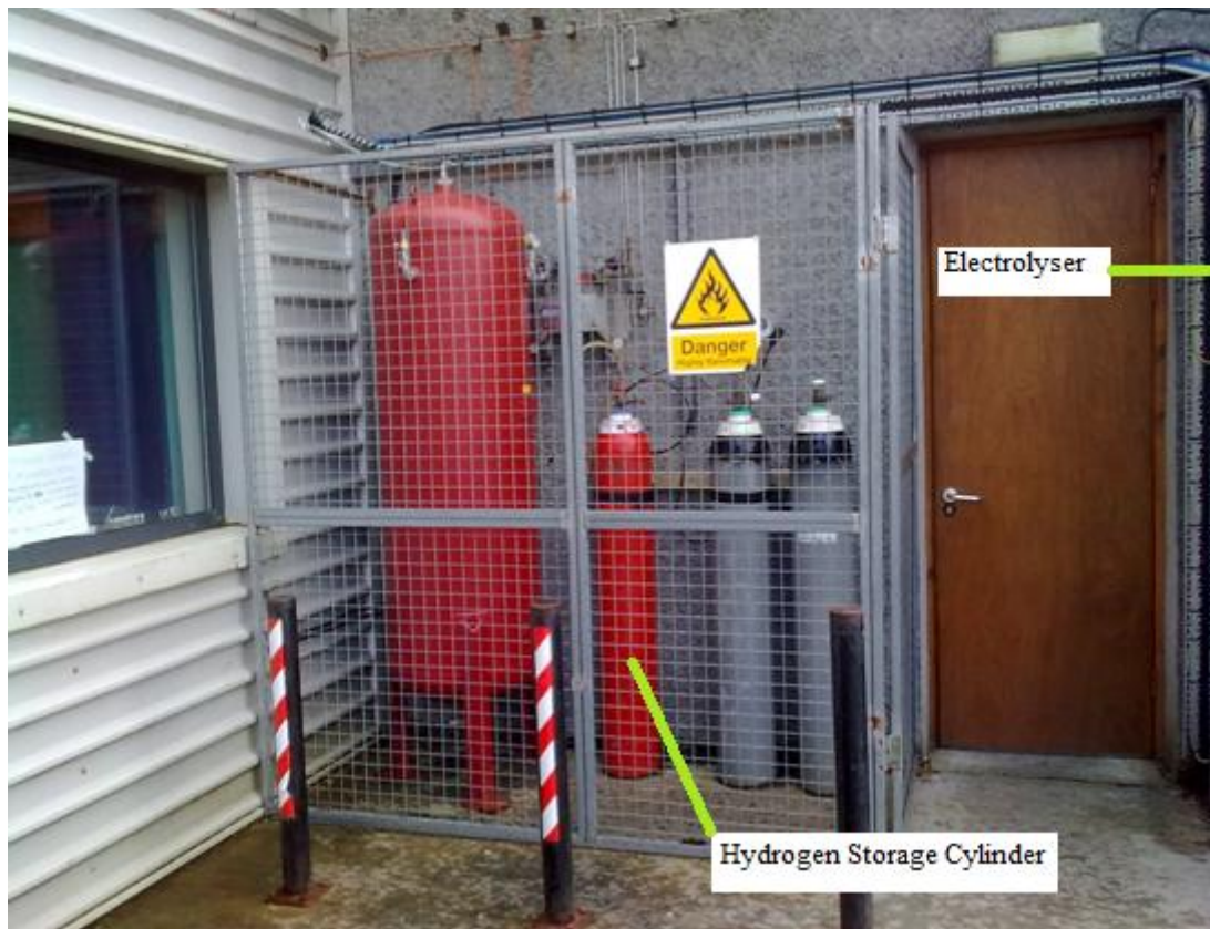
Figure 25 - Hydrogen Storage Tank
