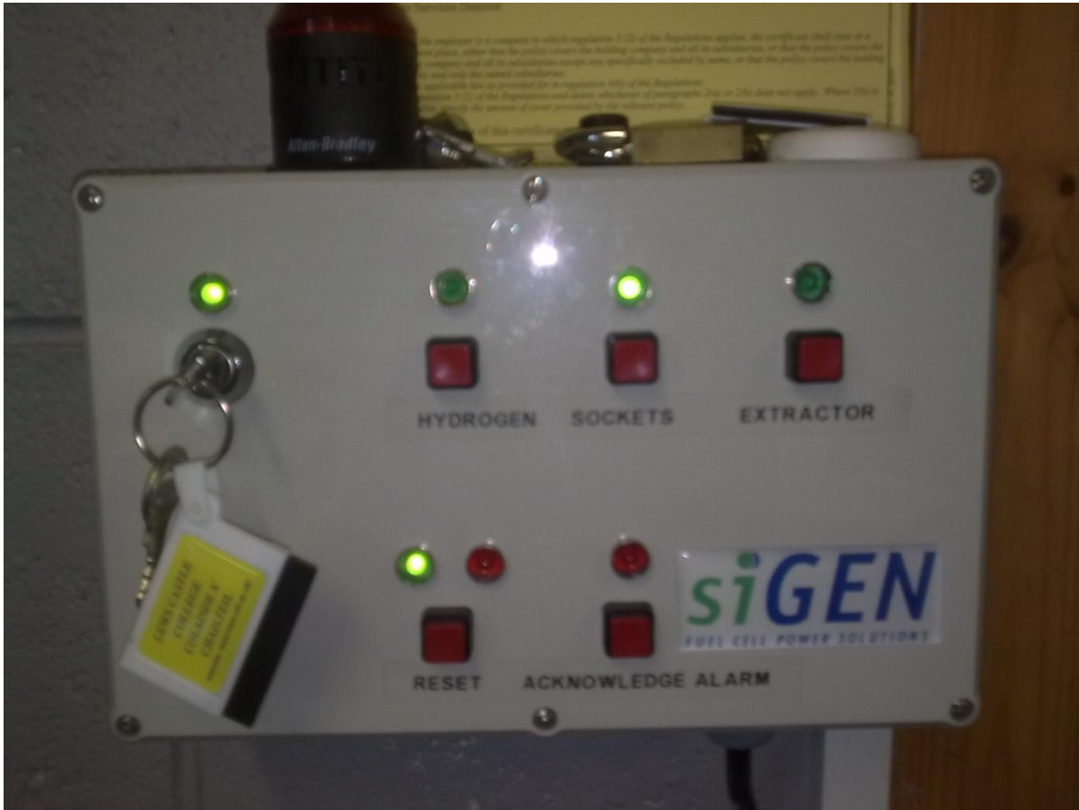
Figure 23 - LCC Hydrogen Laboratory Safety System
