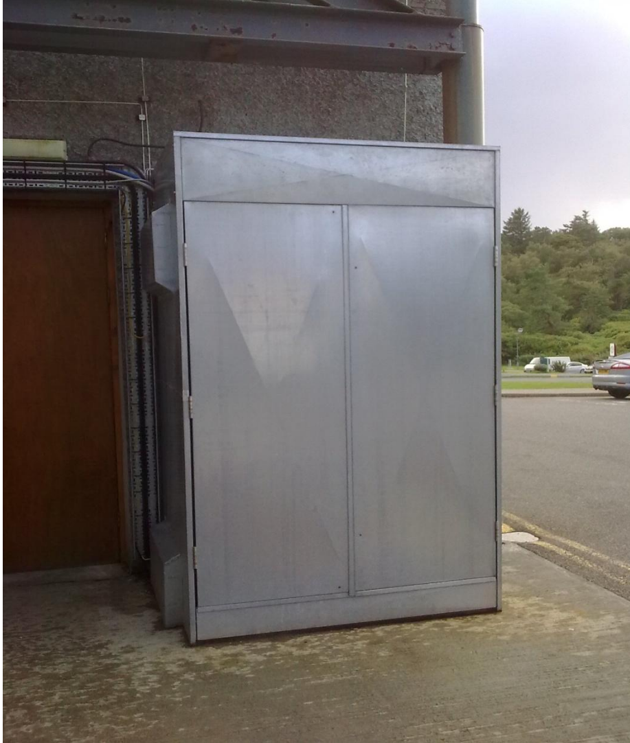
Figure 24 - Electrolyser Containment Unit
