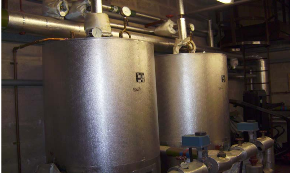
Figure 18: Domestic Hot Water calorifier in Annan Hospital
