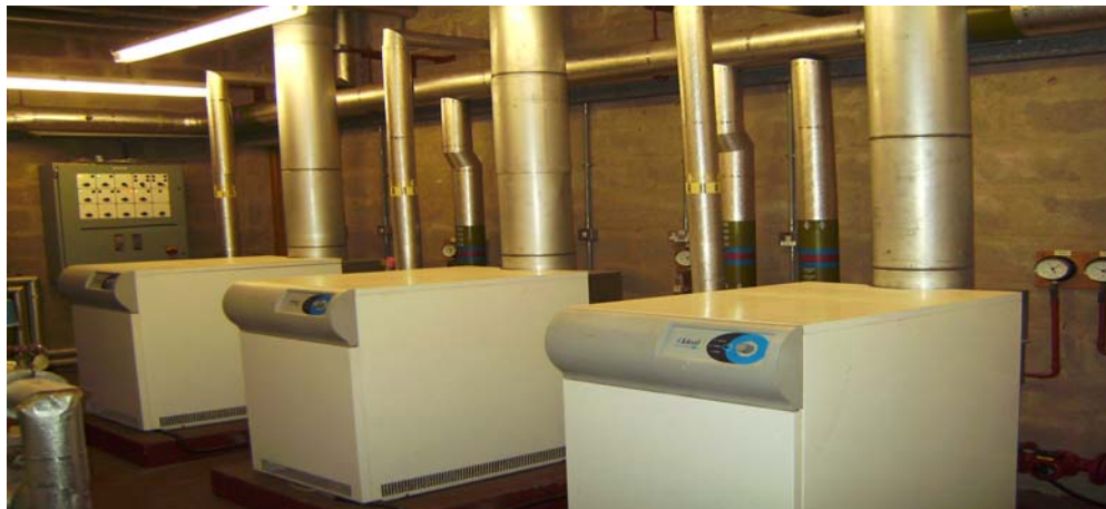
Figure 17: Gas fired unit boilers in Annan hospital
