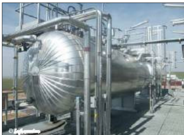
Figure 16- A transesterification reactor. Photo extracted from Infoenviro Caparroso plant report [22]
