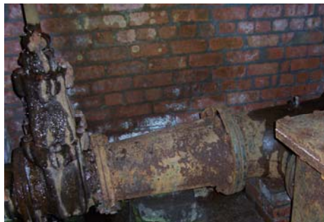
Figure 24: Valve House Pipework
