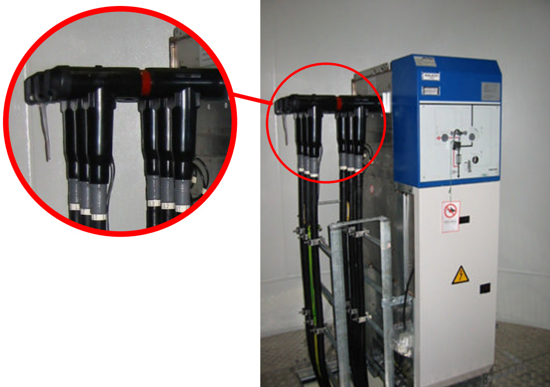
Figure 2.7 Photo of cables terminated to switchgear within a turbine tower [14]
