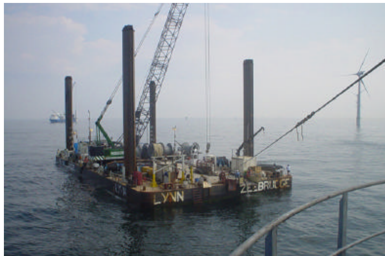
Figure 2.6 Photo of one of the ships used to bury the subsea cables at Horns Rev OWF [14]
