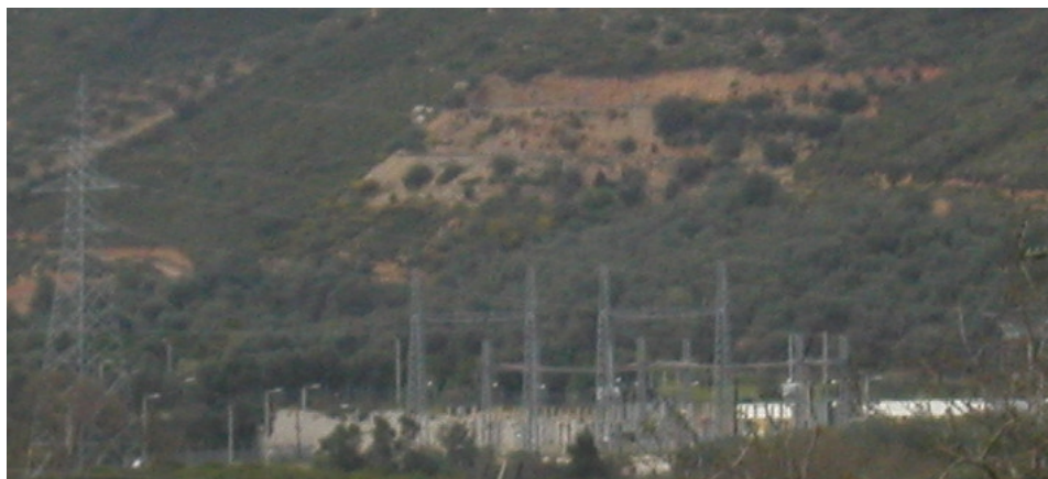
The Substation of Aghia
