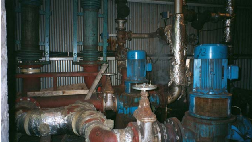
Figure 28 – The Kiln Pumps in the pump room
