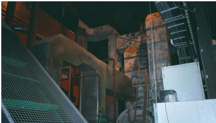
Figure 25 – Furnace (Red) with Boiler on top. The woodfuel conveyer is at the bottom left and some of the ducting is shown.
