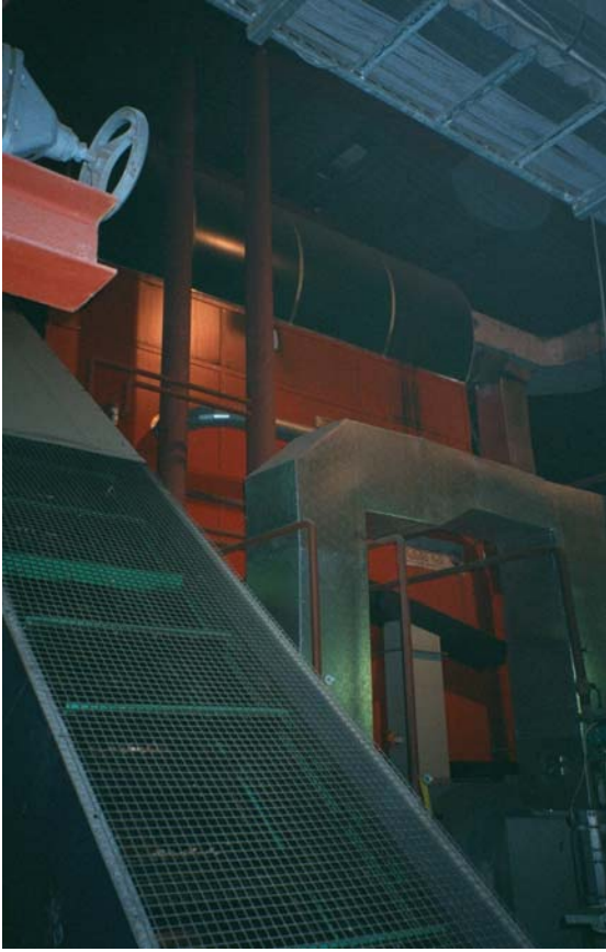
Figure 26 – Closer view of Furnace, Boiler and Woodfuel Conveyor
