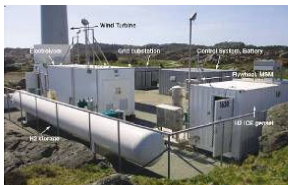
Figure 47: The hydrogen energy system on Utsira Island [44]
