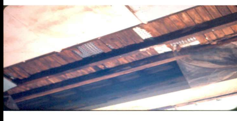
Insulation with vapour decompressing layer below the insulation, interstitial condensation in that layer wetting the timber floor causing rot.
