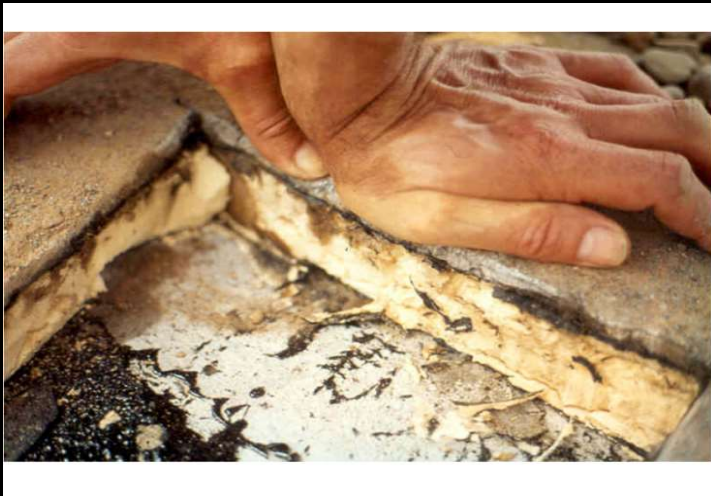
Concrete deck with no vapour retarder. Interstitial condensation wetting the insulation.
