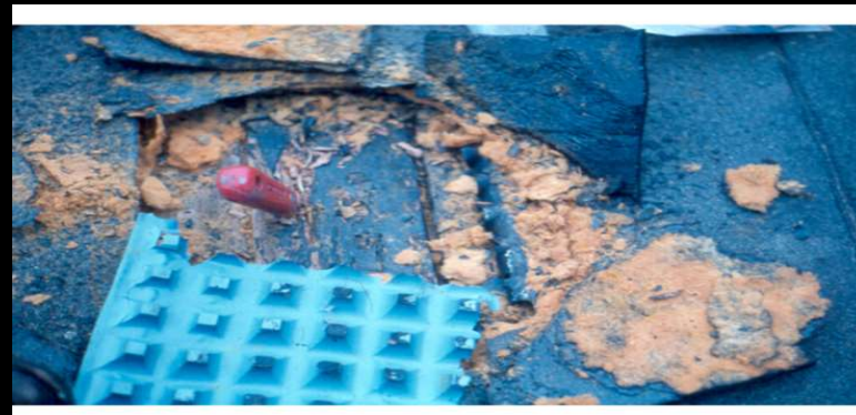
View of the decompressing layer and what is left of the insulation after wetting by interstitial condensation.
